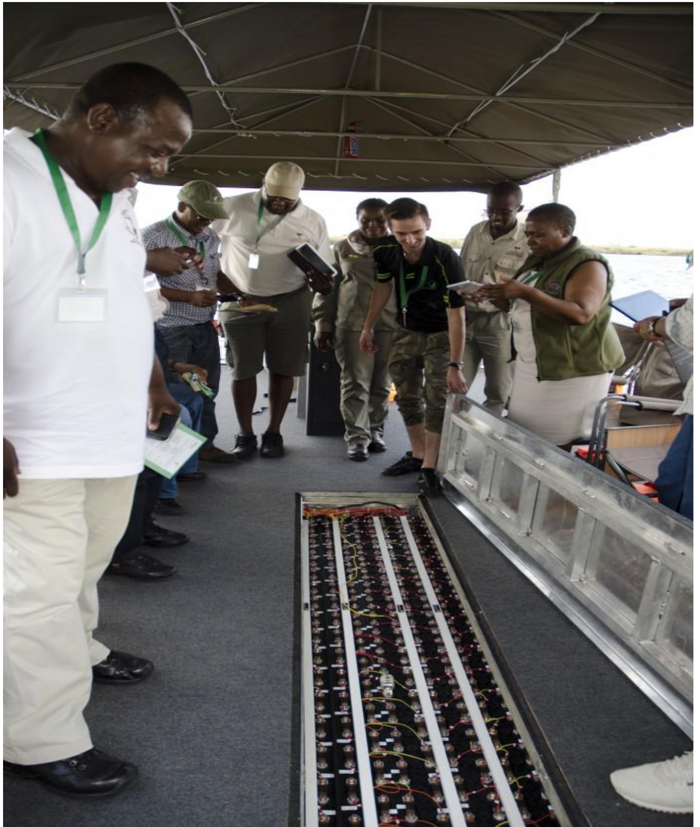
Checking out the lithium battery bank before the first electric safari voyage on the Chobe River
